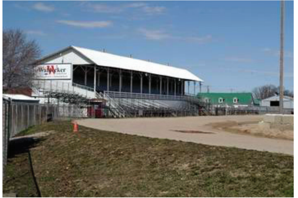
The Grandstand at the Fowlerville Family Fair will be upgraded, thanks to a state grant.
