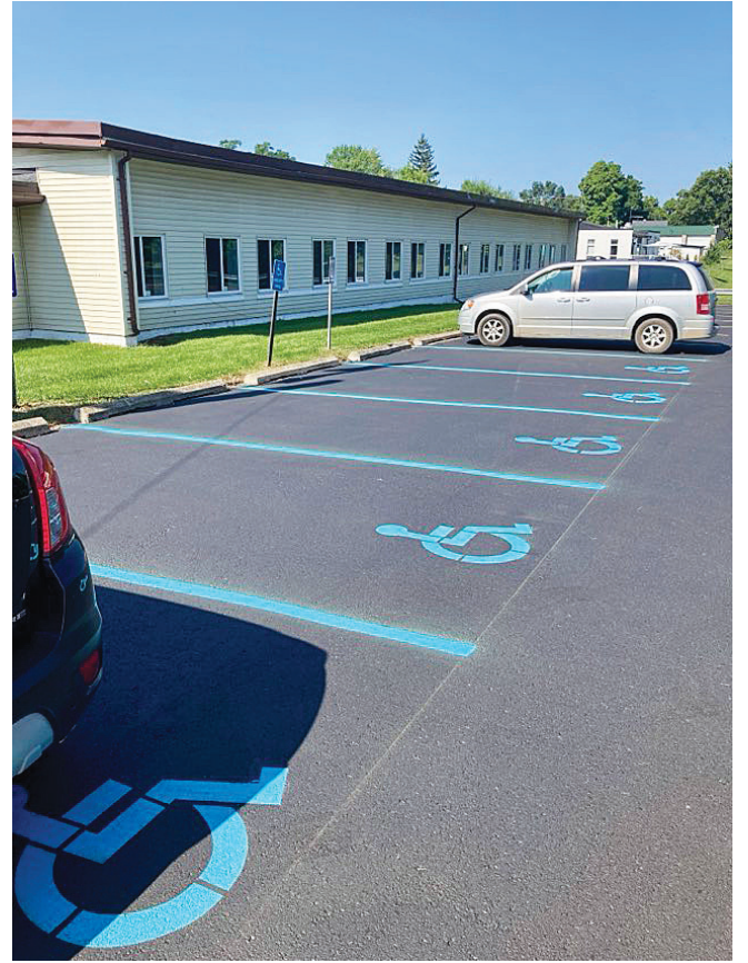
The parking lot was given an upgrade, including crack filling, sealing, and re-stripping.
